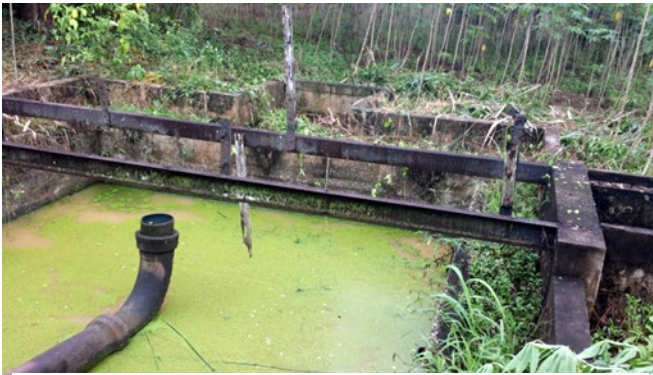
Figure 1.1 Deteriorated wastewater treatment plant at the prison
