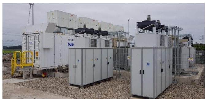
Figuur 4.1 GIGA Rhino battery container on site
